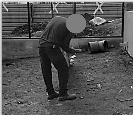
Figure 1. Physical risk: lack of hearing protection. Risk of accident: lack of personal protective equipment: safety glasses and gloves.
