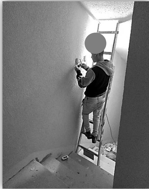
Figure 4. Risk of accident: lack of personal protective equipment (helmet, safety glasses and gloves).
