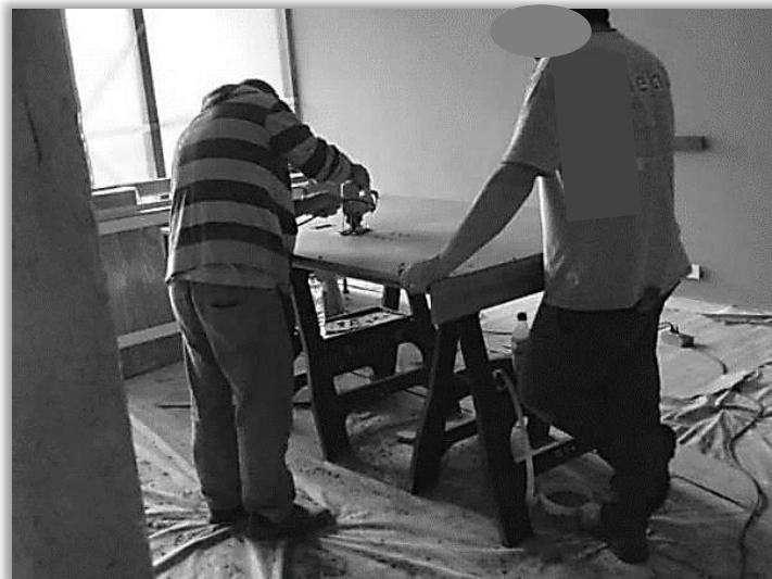
Figure 5. Physical risk: lack of hearing protection. Risk of accident: lack of personal protective equipment (helmet, safety glasses and gloves).
