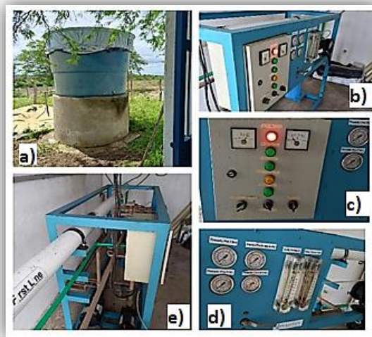
Figure 4. Components of the desalination system at Sítio Telha Branca.
