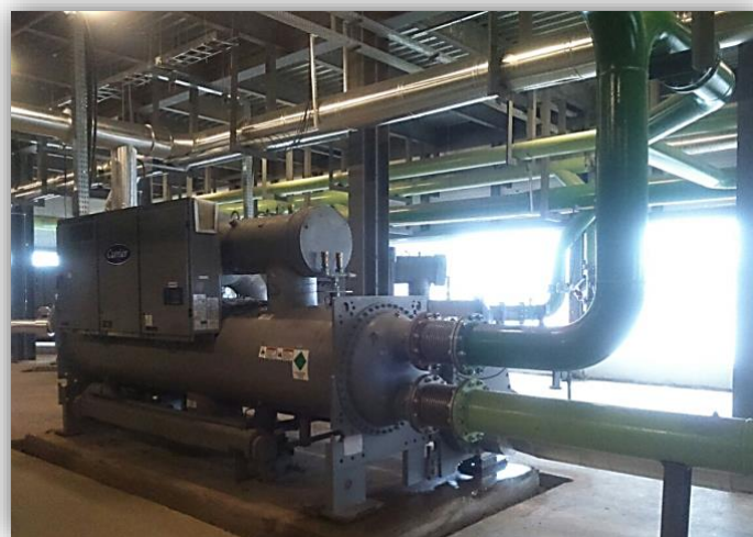
Figure 3. Image of the refrigeration unit used as a model for energy and exergy efficiency study
