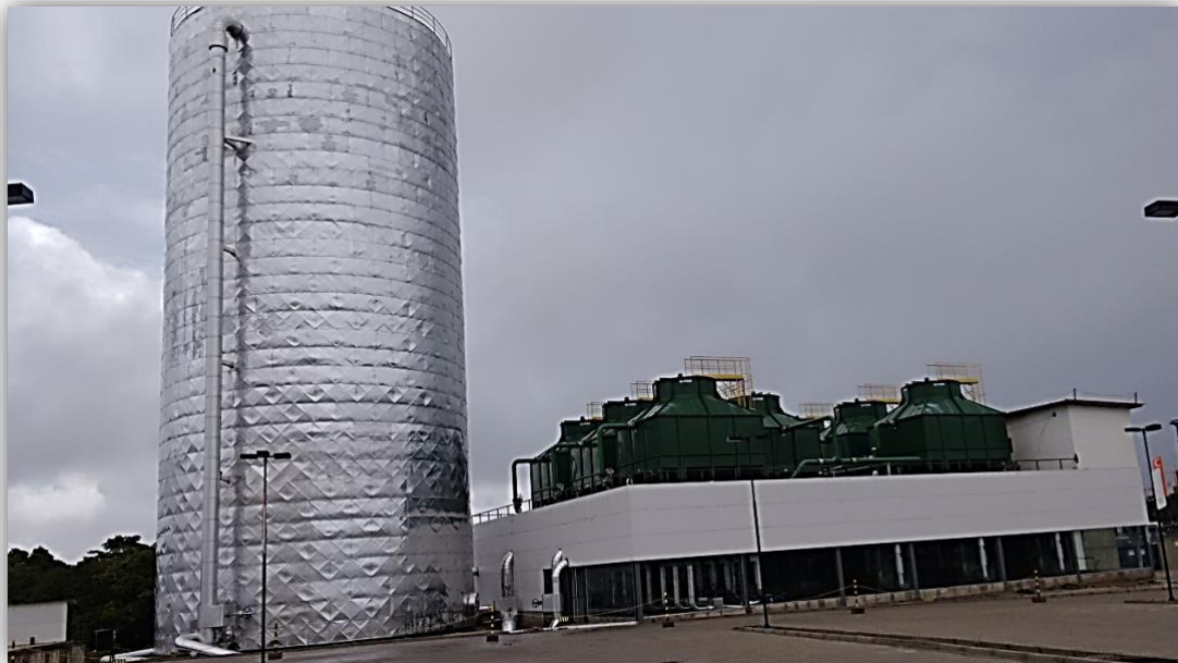
Figure 1. External photo of the Water-Cooled Central where the evaluated equipment is integrated
