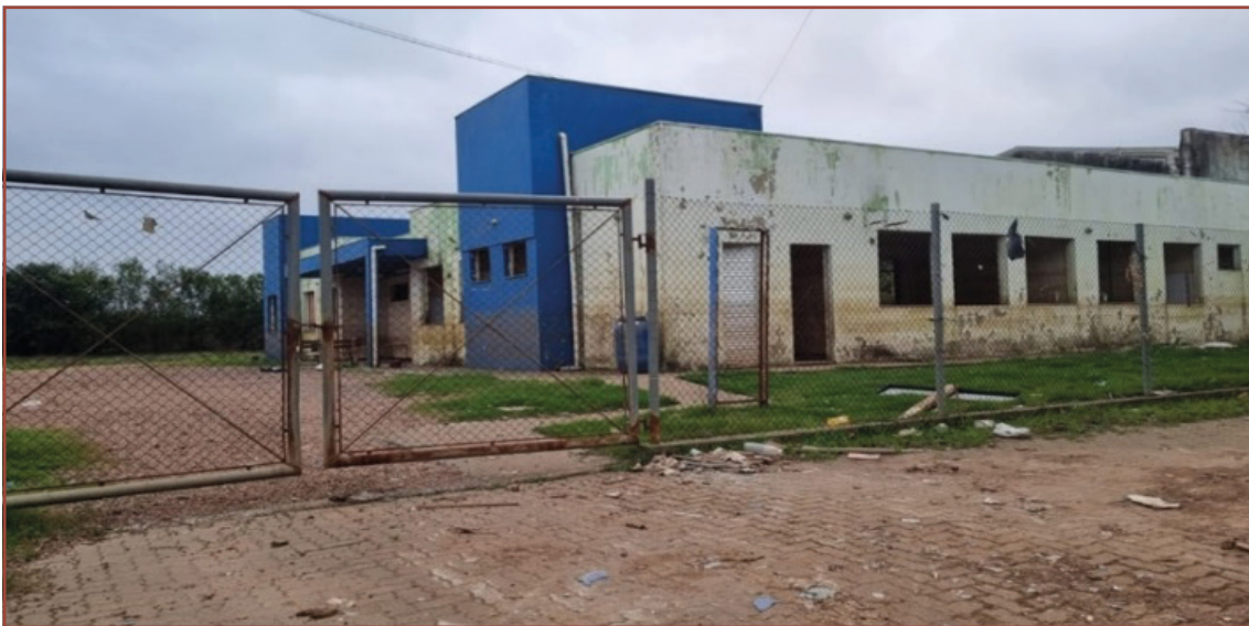
Figure 6 – Primary Health Unit in Eldorado do Sul damaged by flooding
