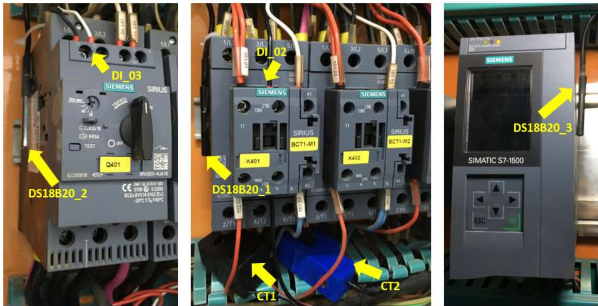
Figure 8. Installation locations for DS18B20 contact temperature sensors, CT1 and CT2 current sensors, and digital inputs for monitoring breaker and contactor status.
